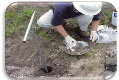
Contractor technicians using hand techniques to determine the extent of soil impacts at the site.
