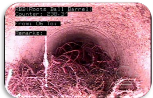
CCTV image of interior pipe obstruction
