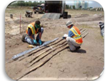
Field staff used direct push technology (DPT) to evaluate chlorinated solvent mass partitioning at finite intervals in the subsurface.
