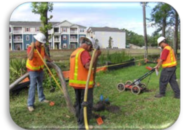
Ground penetrating radar and test hole excavations are used to locate, identify, and verify utility locations and provide a means for elevation surveys of key subsurface features.
