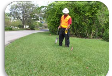
Field crews use a wide range of prospecting tools to locate underground utilities.
