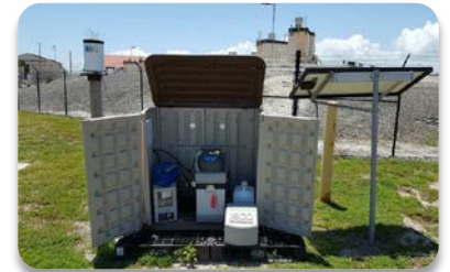
Monitoring stations were designed, installed, and maintained by the project team.
